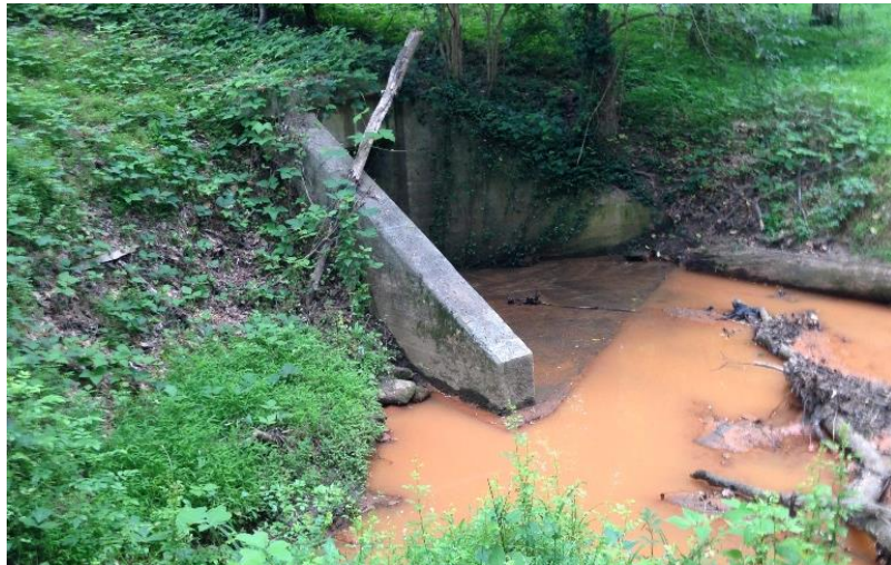
Existing Stream has excess sediment, particularly in 'Pod 3'
